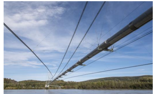
Above-Ground Pipeline Crossing
